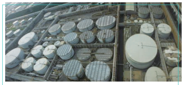
Wastewater treatment plant (After improvement)
